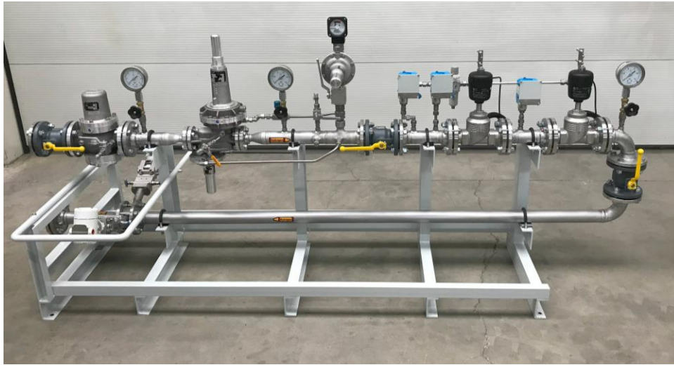
Gas safety station
