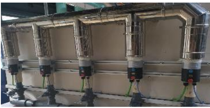
500 kW air heater (up to 600 °C)
