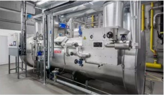
Waste heat recovery boilers
